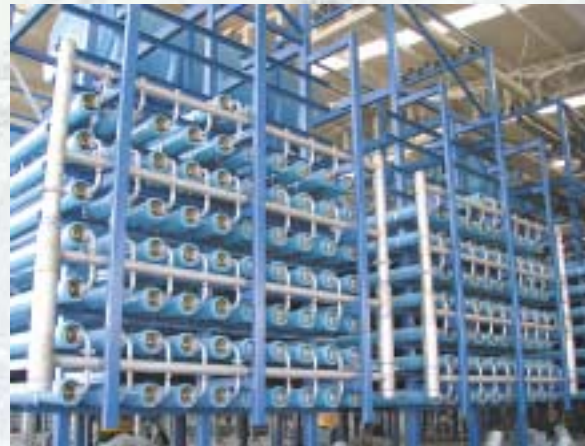
SWC installation at Carboneras, Spain
